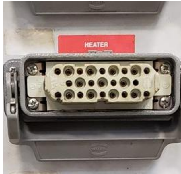
Pushed Back Inserts High Amp Deterioration (10-amp rating)
